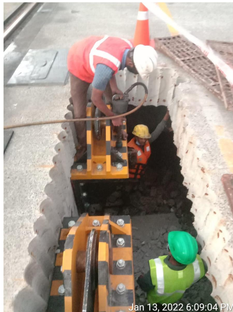
Adani Port – Anchor Tie down
